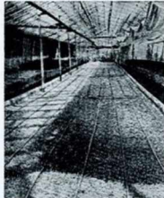
Heating cable installed in a greenhouse bench
